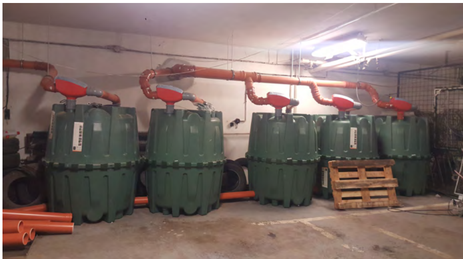
Water tanks in the basement of the City Municipality building, collecting the rainwater, which is afterwards used for flushing lavatories, Zvolen, Slovakia (Photo: Maria Bihunova)
