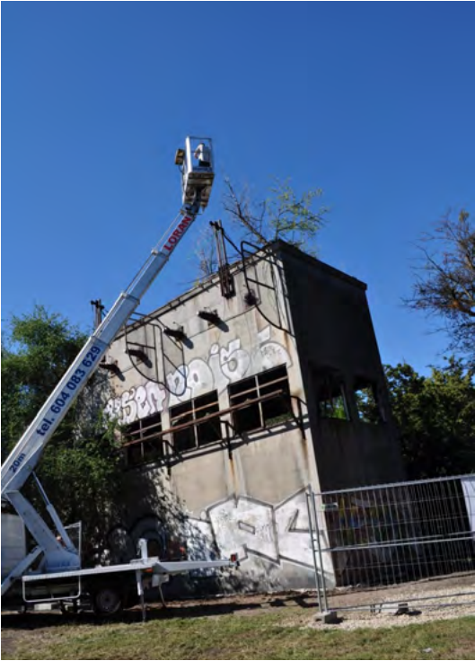
Transformer station building, Niskie Łąki estate in Wrocław, Poland (Photo: Marta Weber-Siwirska)
